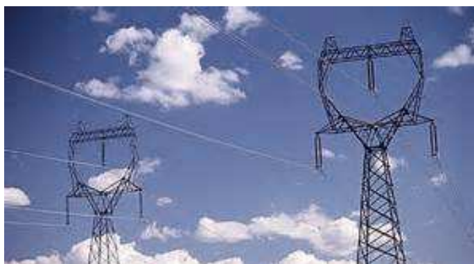
FIGURE 4.7 – Des poteaux ERDF.
