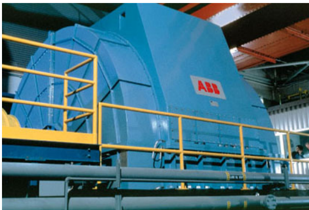
New 100-MW (135,000-HP) synchronous motor used to operate the NTF wind tunnel
